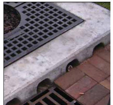
Outlets blocked by other features
