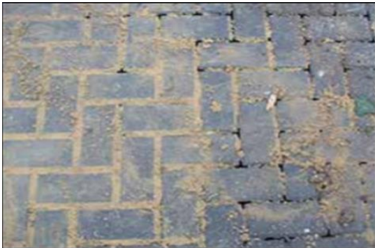
Blocked permeable paving
